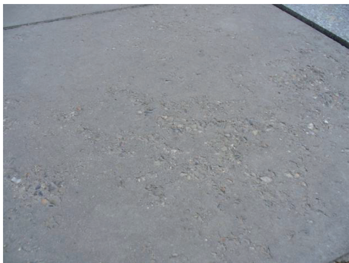
Fig. 1. Two years old concrete slab, damaged by scaling. (Prague)
